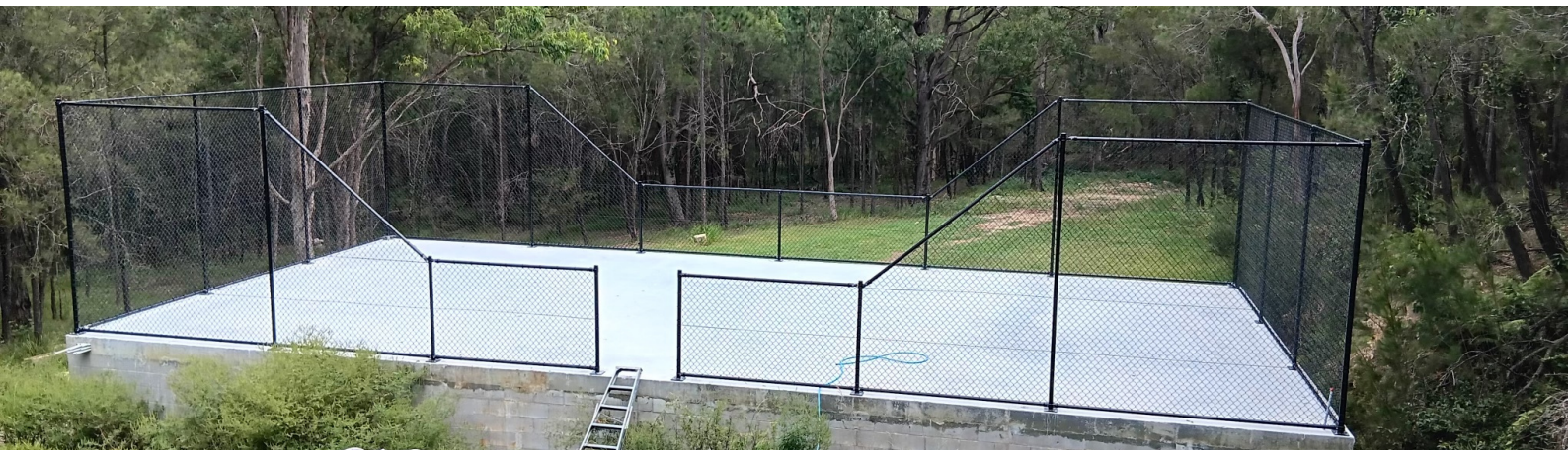
Mini tennis court on a suspended slab with diagonal rails transitioning from 3000mm high to 1200mm high
