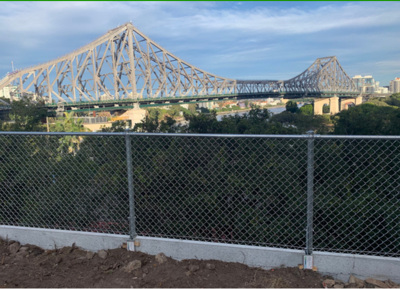
1200mm high galvanised chainwire with top rail mounted on to concrete sleeper wall
